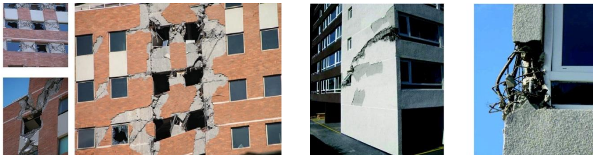
Figure 3 : Performance of reinforced concrete buildings during Chile earthquake.
