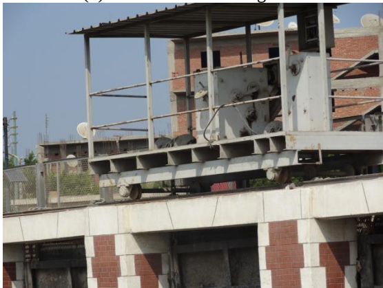
Photo (5): Gate lifting system
