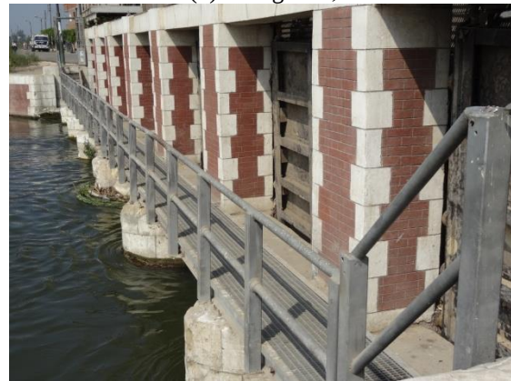
Photo (6): Regulator gates
