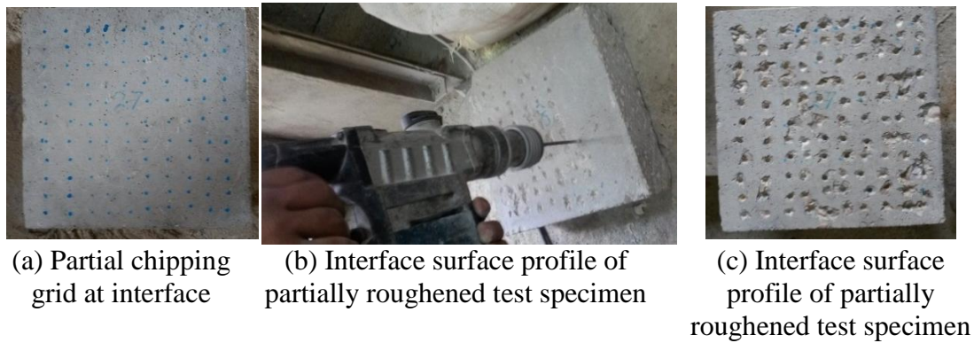
Figure (4): Partial chipping of test specimens
